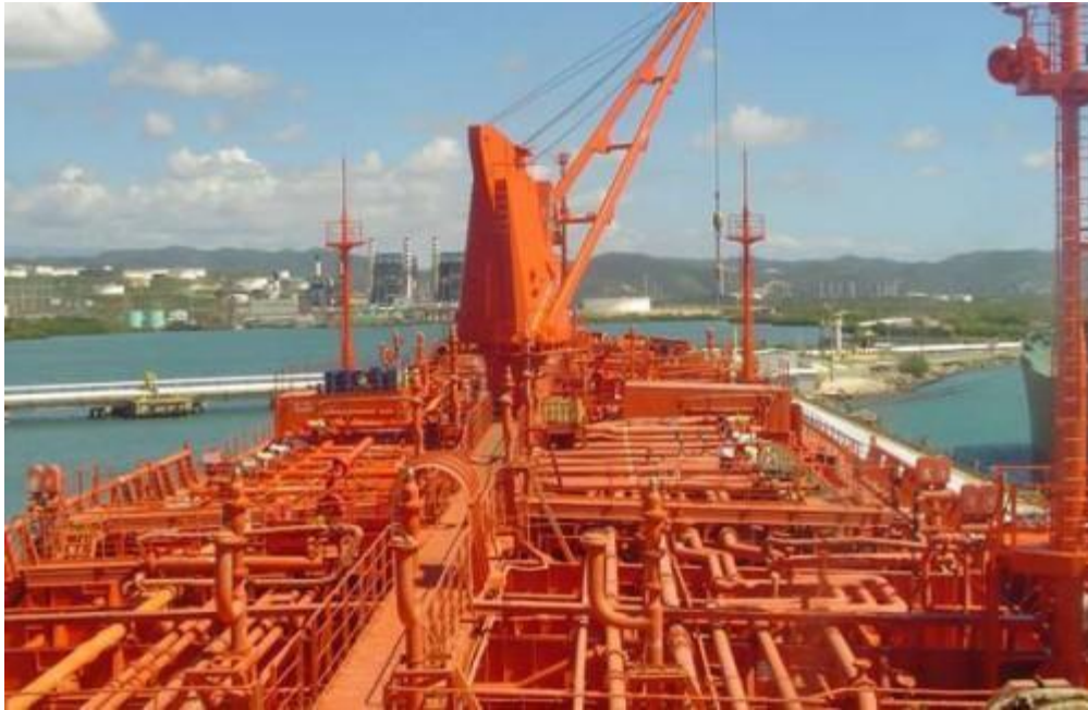
Fig. 4.2.5.A : Chemical tanker cargo pipelines
